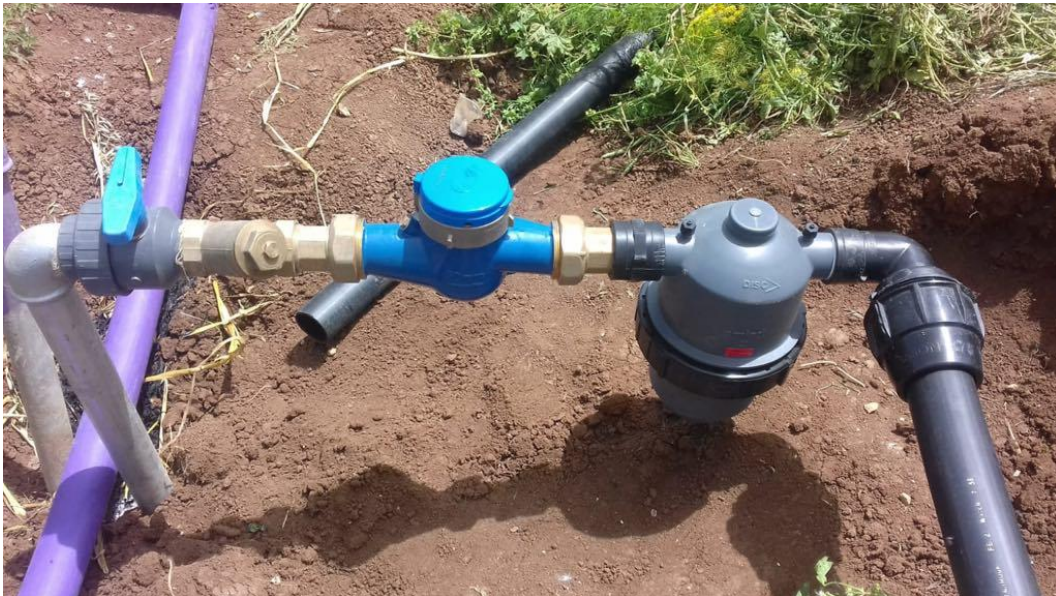
Figure 3.3: TWW filtration by disc filter at gate valve
